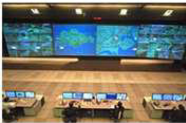
Operation Control Center
