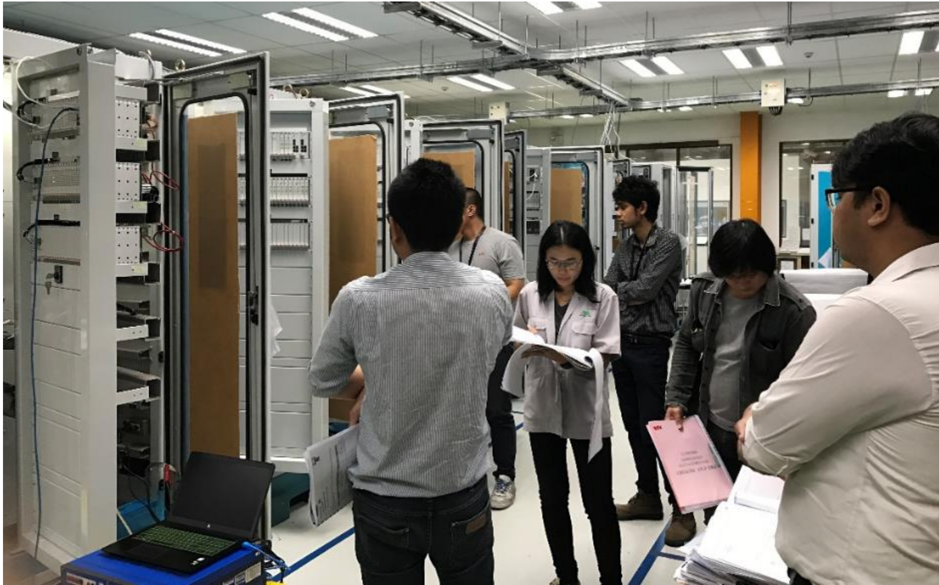
SCADA - Remote Terminal Unit (RTU)
