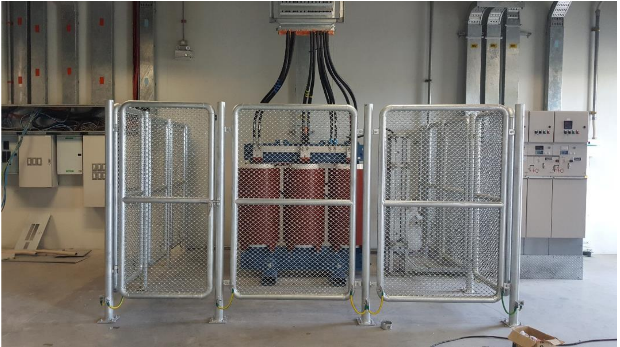
Power Supply – Service Transformer at OCC
