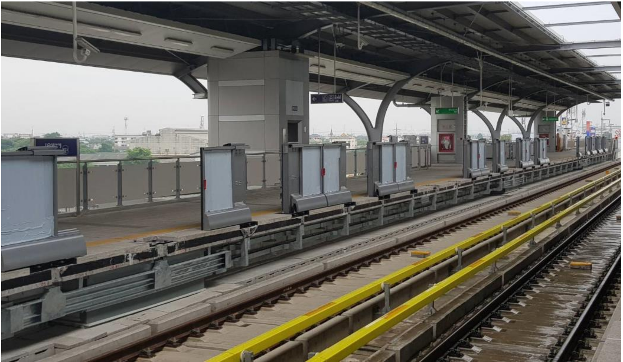
Platform Screen Door at Station E23
