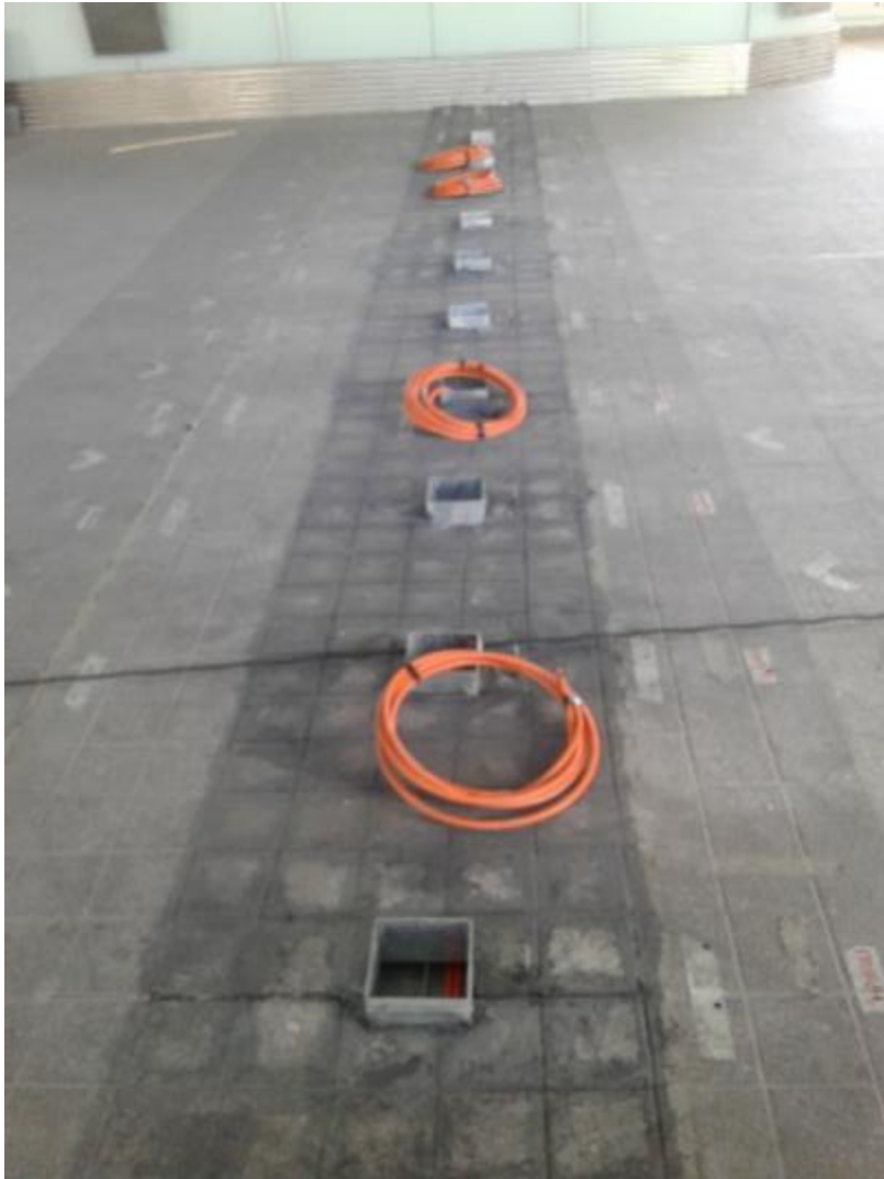
Automatic Fare Collection – Installation at Station E19
