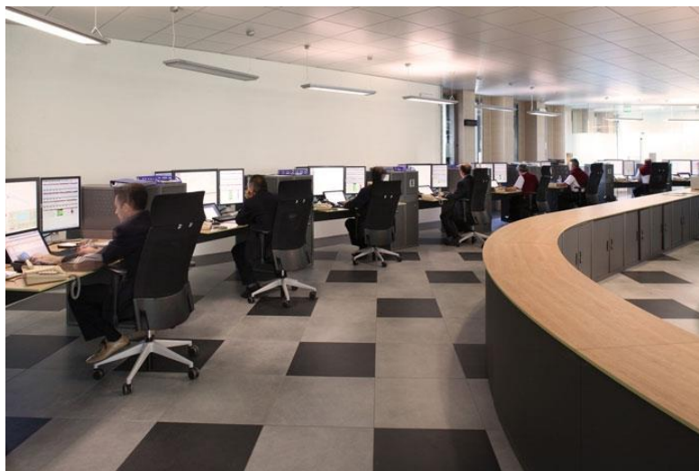
Figure 7-69 ATM Transport Management Control Room
