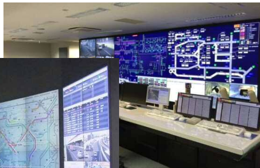
Facilities control system
