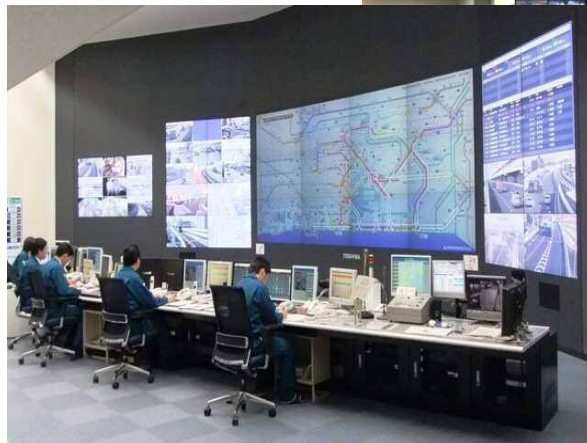
Traffic control system
